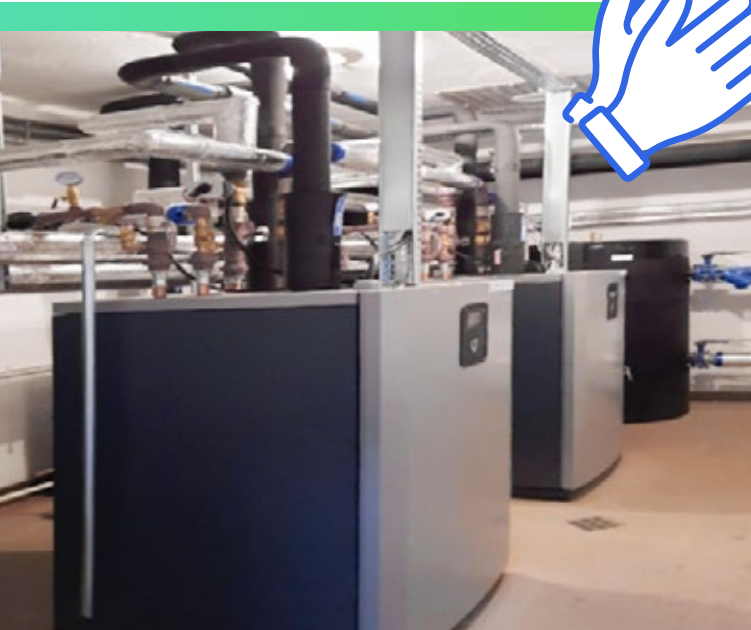
Heating pumps in Oleśnica, Poland
